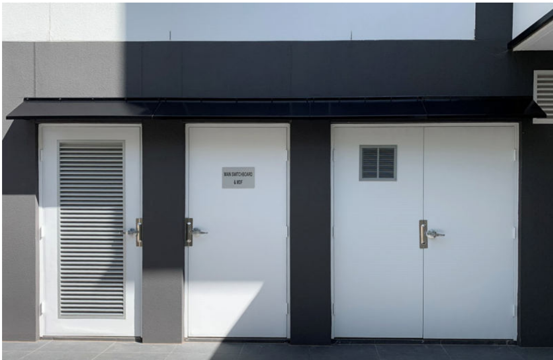
An example of how louvre blades can be inserted into a door of an electrical cupboard to allow ventilation
